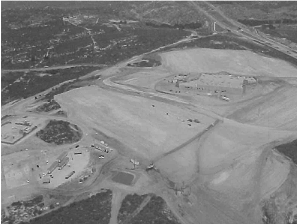
Plate 33: View of the construction/grading activities associated with the Casino/Travel Center on the Campo Indian Reservation looking northwest.
